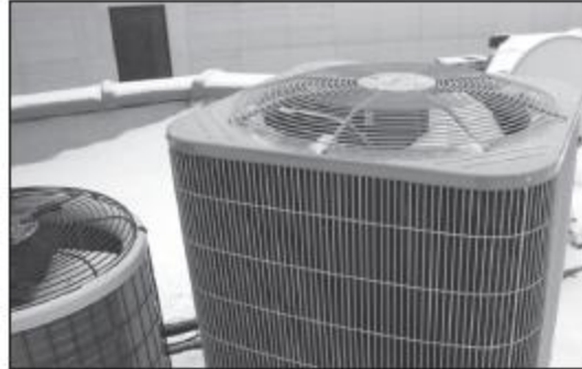
Air conditioning systems
