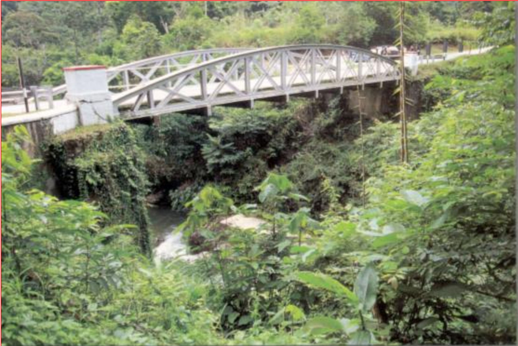
This 24m span steel arch bridge is on Federal Route 55 leading to Fraser's Hill. The deck was constructed using steel beam with buckle plate. The bridge was built in 1950.
