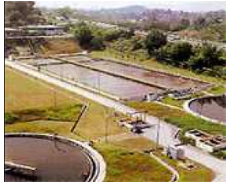
Activated sludge plant
