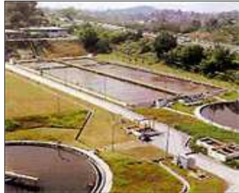
Activated sludge plant
